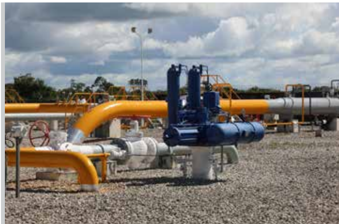
Somangafungu gas receiving station
